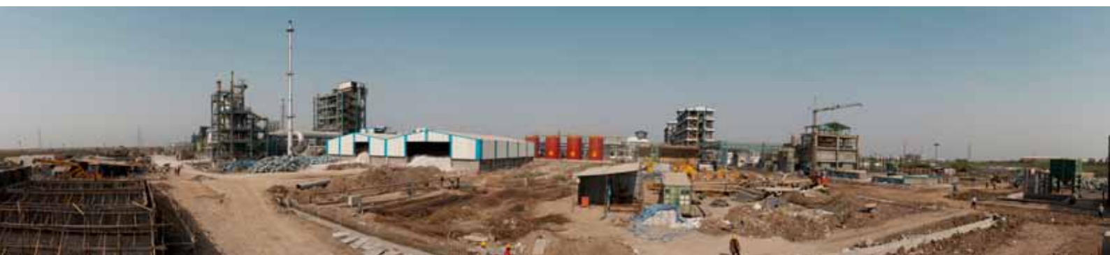
A view of ongoing expansion projects at the SRF Chemicals Complex, Dahej, Gujarat
